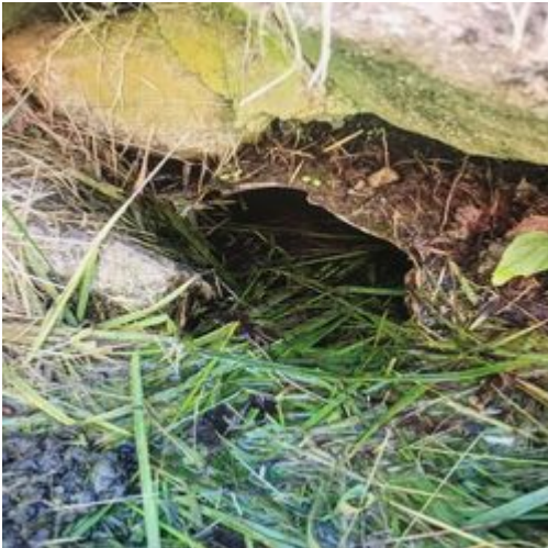
Outfall 37 filled with stagnant water/buried
